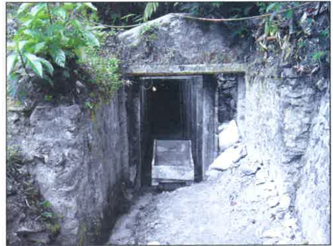
Figure 3. An adit used by local gold miners for extracting gold ore at Cineam area.
